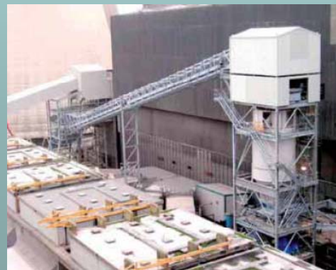
Fiddlers Ferry, UK – 20% biomass + 80% coal
